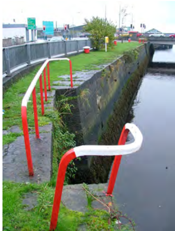
Old Quay Walls - Suggested removal of existing barrier with re-design and replacement with more aesthetically pleasing railings.
